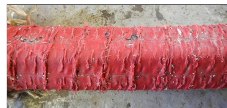
Figure 10: Anti-friction screen showing evidence of pressure tears and wear. Bio-fouling debris is also viable.
